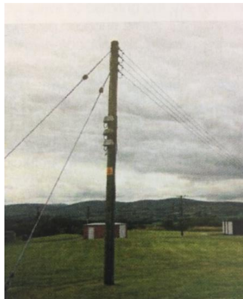
400v distribution line
