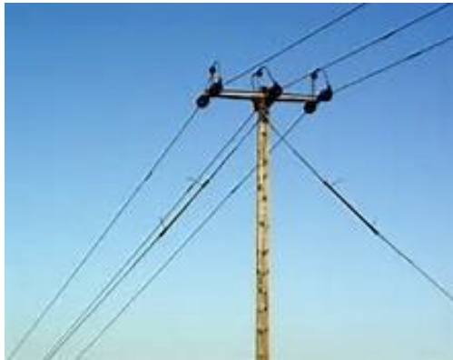
Wooden poles (11kV and 33kV)
