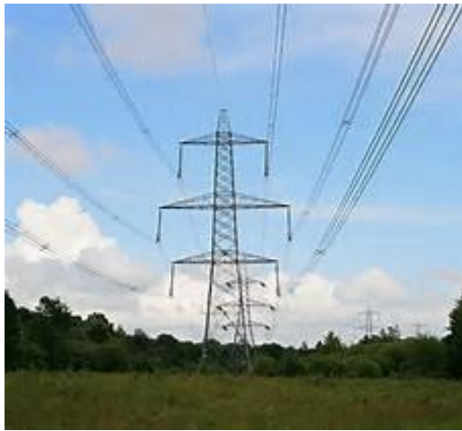
The largest steel pylons (275kV and 400kV)
