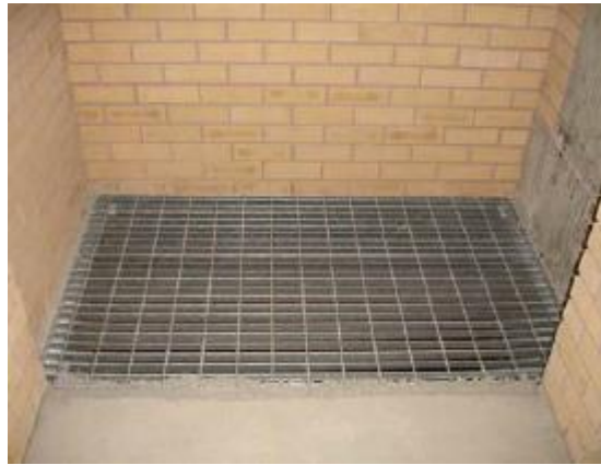
Secure cover over riser opening
