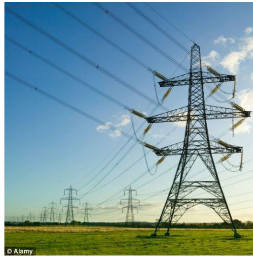
Smaller steel pylons (132kV)
